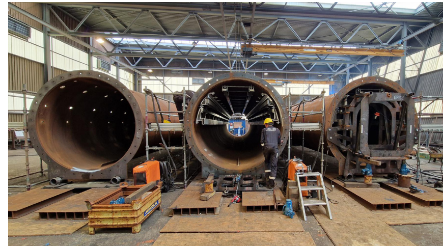
Figure 29: The assembly of guideway tracks and internals using an assembly jig at Mercon in Gorinchem.
